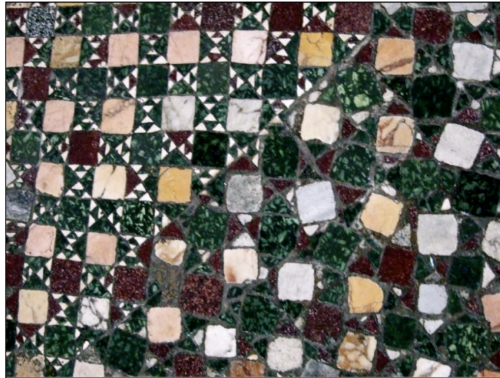
Figure 7.1: Floor in (dis)repair in San Lorenzo fuori le Mura. Photo by Norman
